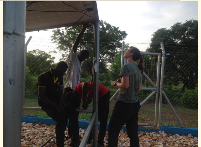
Relocation of the solar pump's sun sensor
