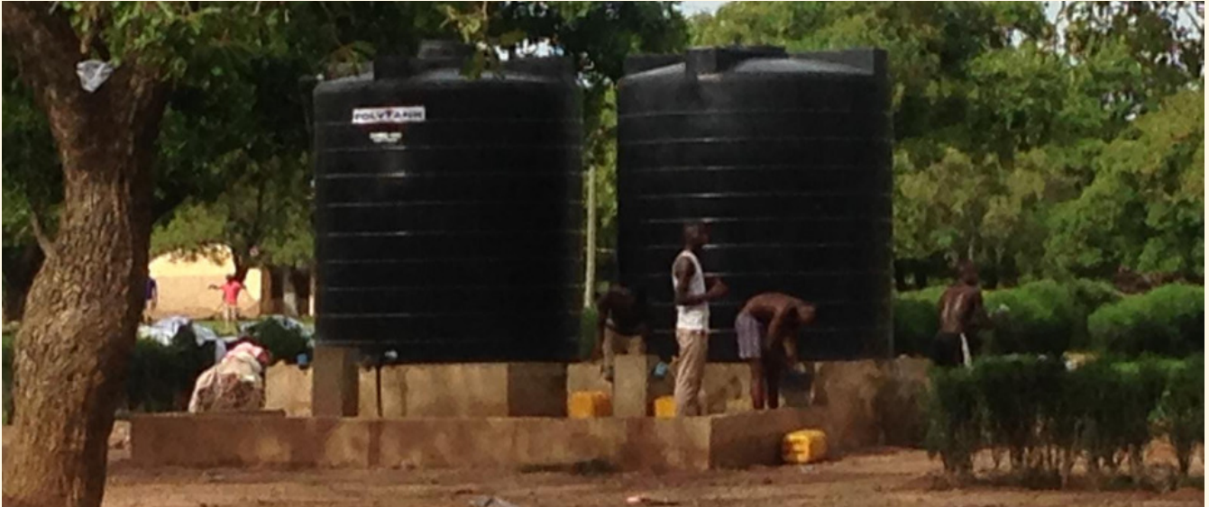
The water distribution system being used at the boys dormitory
