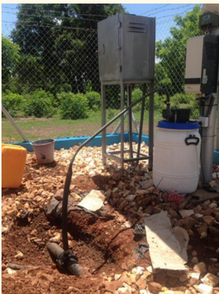
Chlorine pump operating properly with new valve!
